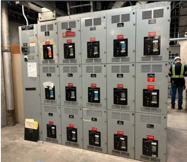
Fig. 4 480V Fused Metal Enclosed Switchgear (Used with permission from Author)
