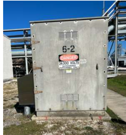
Fig. 3 24kV Aboveground Junction Box (Used with permission from the Author)
