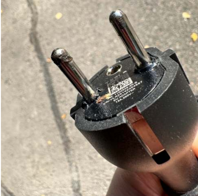
Fig. 3 An overheated Schuko (Type F) plug in a Mode 2 electric vehicle charging cable. Signs of rapid overheating can be seen in the plastic parts, as well as overheating and arcing marks in the conductive parts.
