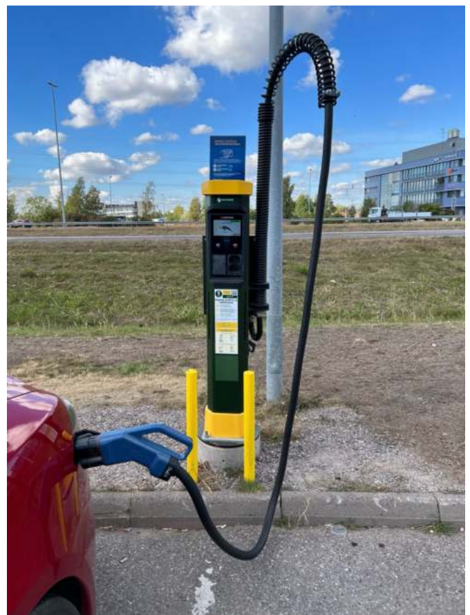
Fig. 6 An example of a cable management solution which decreases the likelihood of the cable being driven over or getting looped around the tow hitch of the vehicle.
